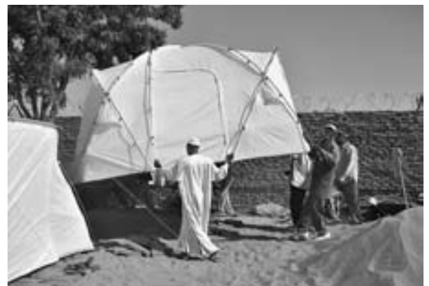
Setting up tents to accommodate staff while permanent houses are under construction in the LWF/ACT compound in Koukou. © NCA/ACT International/B. Rödland
