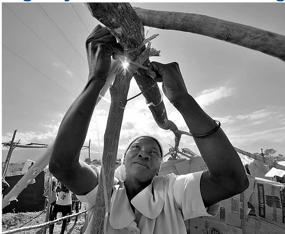
A woman builds a temporary home in a camp north of the Haitian capital Port-au-Prince. The LWF provided rain-proof shelter for Haitians who lost their homes in the 12 January earthquake. © Paul Jeffrey/ACT Alliance
