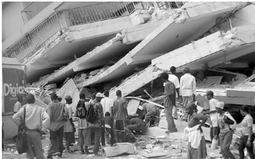
This is what remained of a hospital building in Haiti’s capital Port-au-Prince after the 12 January earthquake. © DCA/ACT Alliance
