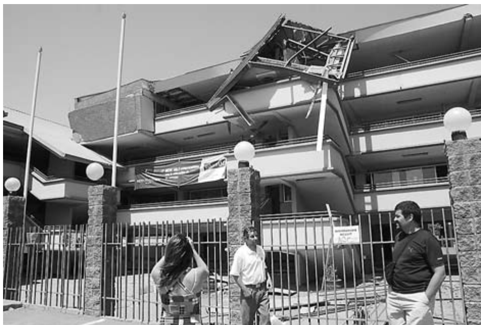
An earthquake-damaged building in the city of Maipú, central Chile © Pablo Ordenes/flickr
