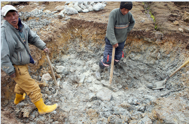
In Altarani, the process of building a new water pipe for the village is well underway with local people digging holes for the trench. Photo: LWF/I. Dorji
