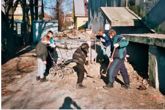
During 1998-2000, the children carried more than 230 m 3 of building refuse out of the church and church basement. Photo: Center for Pastoral Care
